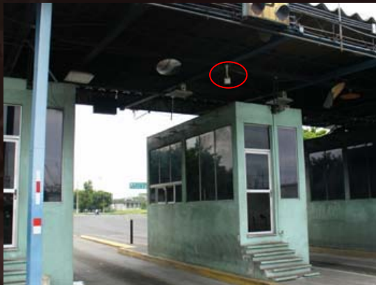
Fixed Reader at gate of Puerto Quetzal, Guatemala
